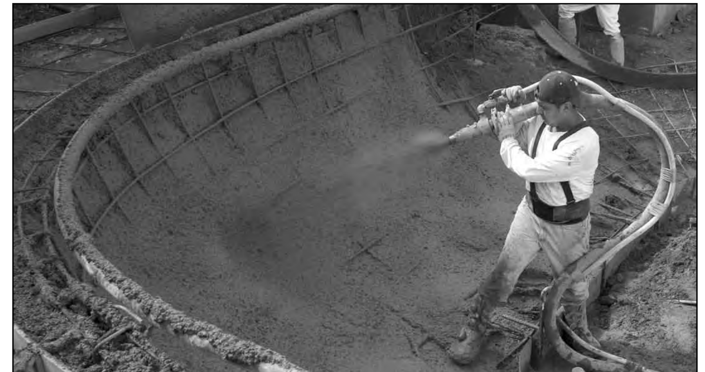
The best skatepark design can go astray without critical oversight by experienced personnel during construction. A skatepark consultant should be involved throughout the process.
